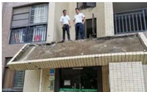
悬挑雨棚坍塌
